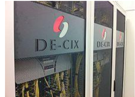
A 19-inch rack used for switches at the DE-CIX in Frankfurt, Germany
